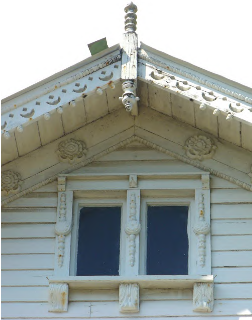
FIGURE 27: SKYLIGHT, WOOD GABLE POST, ORNAMENTAL TURNED BOSSES AND PIERCED BARGEBOARD DETAIL ON A HISTORIC GEORGETOWN HOUSE
